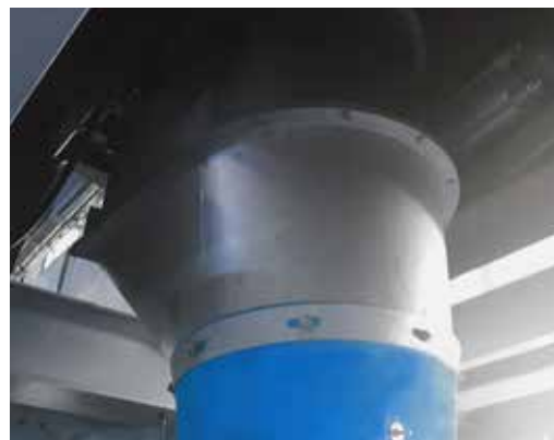
External view: Discharge area and transfer pipe
